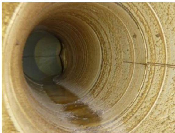
Without ozone cleaning system
