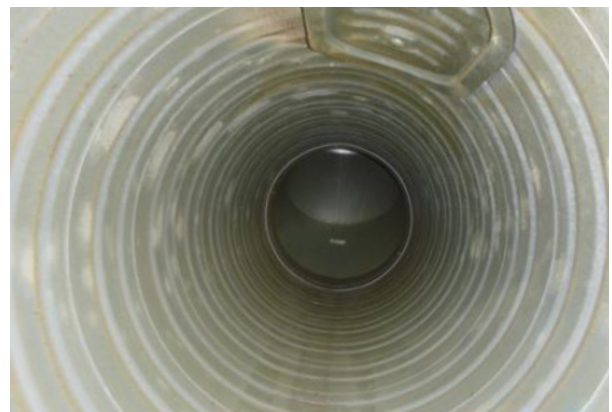
Exhaust duct with ozone cleaning system
