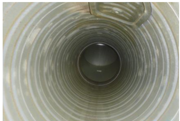
Exhaust duct with ozone cleaning system
