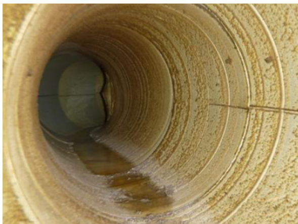
Exhaust duct without ozone cleaning system
