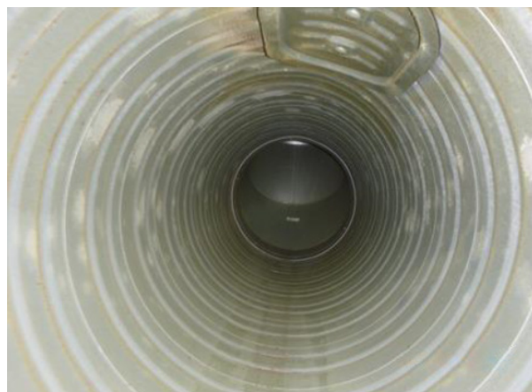
Exhaust duct with ozone cleaning system
