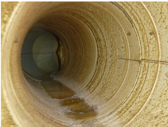
Without ozone cleaning system
