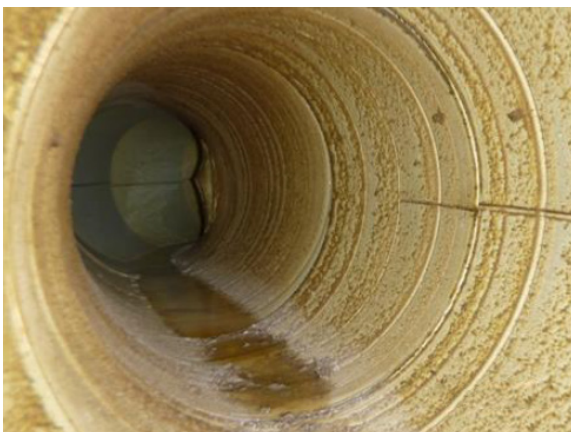
Without ozone cleaning system
